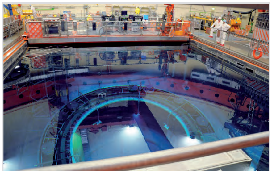
Fig. 7: View of the upper reactor pressure vessel in the containment building during maintenance. (Photo: NPP Leibstadt, Switzerland)
