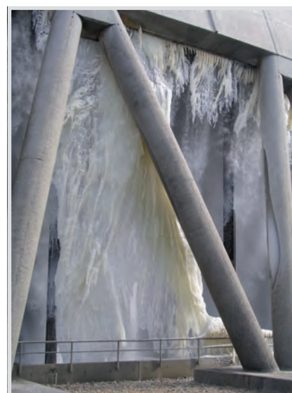
Fig. 8: Cooling tower in winter.
