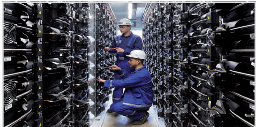
Fig. 10: STEAG large-scale storage battery Source: STEAG
