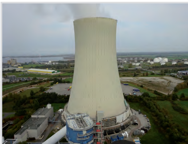
Fig. 7: Cooling tower of the thermal power plant Rostock under revision, KNG.
