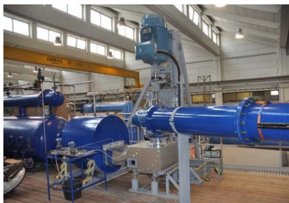
Experimental setup and measurements at the test rig
