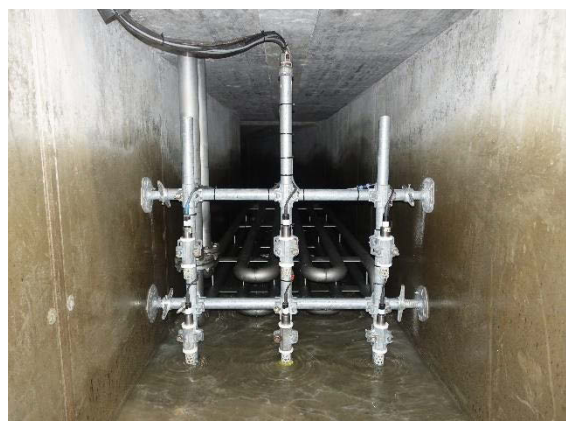
Low pressure measuring section at HPP Tannuwald, ALPIQ, Switzerland.
