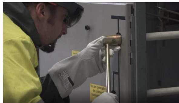
Switching operations in a medium-voltage network.
