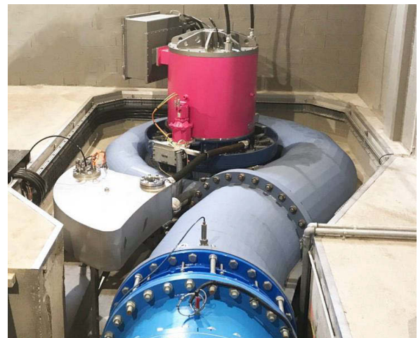
Medium head DIVE-Turbine in France. Installed capacity 600 kW.
