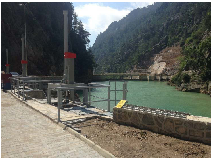
HPP Dagbasi (Turkey): Control for hydropower plant and cloud integration
