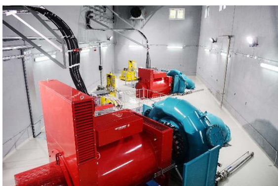
Machine room in Zapeče, Bosnia.
