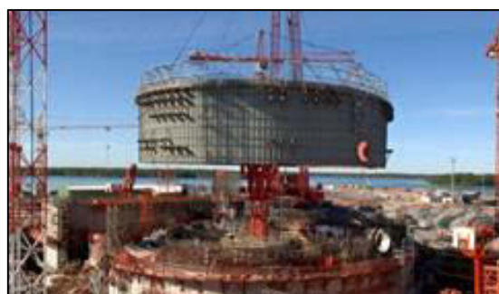
Nuclear Power Plant, Containment Liner (at that time under construction); © Babcock Noell GmbH (nowadays Bilfinger Noell).
