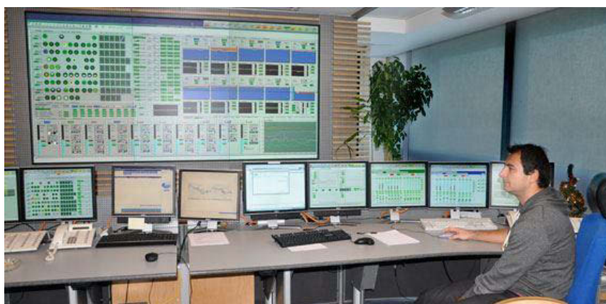
In VHP's central control room at the HPP Freudenu close to Vienna, the 10 HPP located along the Austrian section of river Danube are managed. VHP's training system utilizes VIRTUAL RIVER as a substitute for the real river.
