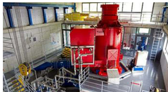
Project Schattenhalb: Synchronous generator for a Pelton Turbine.
