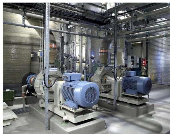
Oxyfuel Pilot Plant; © Babcock Noell GmbH (nowadays Bilfinger Noell).
