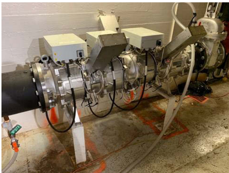
Atlantium's Hydro-Optic™ (HOD) UV demonstration unit installed at OPG DeCew II Generating Station.
